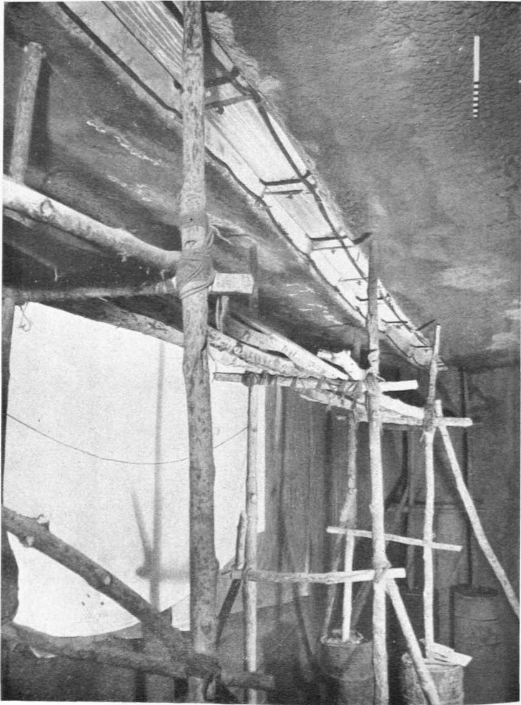
Ajanta: Cave I, provision of ceiling-drain. See page 45
